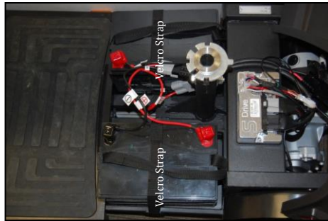
Figure 17. Installation des batteries
